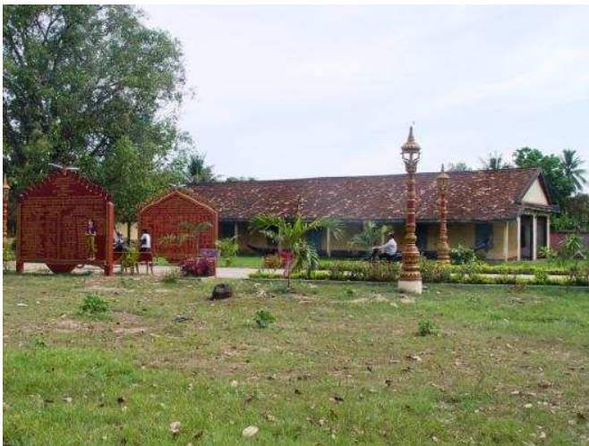
The old school building, with leaky roof.
